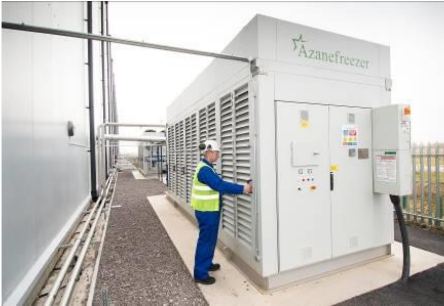
Caption: Thanks to the intelligent system design of the Azanefreezer by Star Refrigeration Ltd., it was possible to reduce the ammonia charge at Farmfoods to 0.1 kg per kW.
